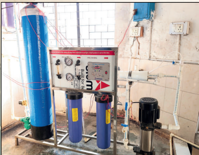
RO Plant (BAK Hostel)
