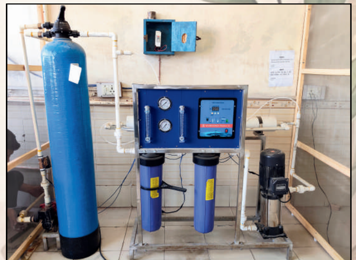
RO Plant (Bi Amma Hostel)
